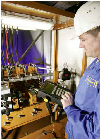
Service Hydraulikanlage Service hydraulic unit
